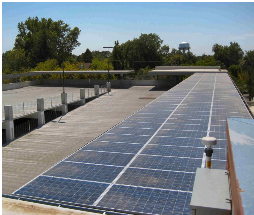
Figure 5. 78 kWdc PV array on Normal Avenue Parking Structure.
