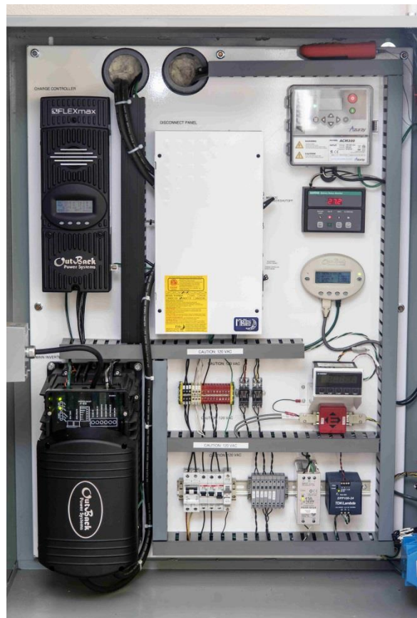
Figure 3. PV electrical components.
