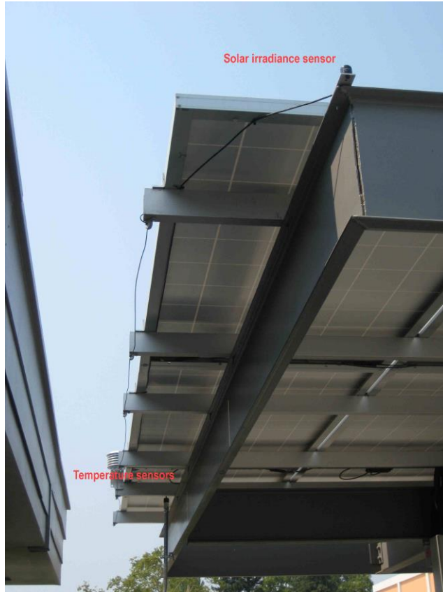
Figure 6. Installed weather station sensors.
